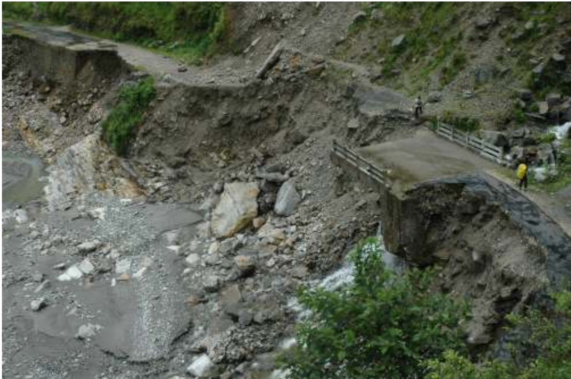
Figure 17: A destroyed road and bridge between Bungapani and Umargada
